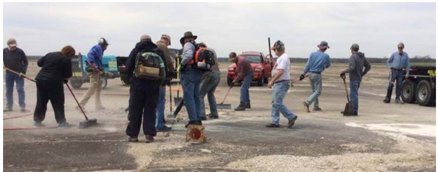
The Dig Party Crew goes at it to repair the autocross course.
